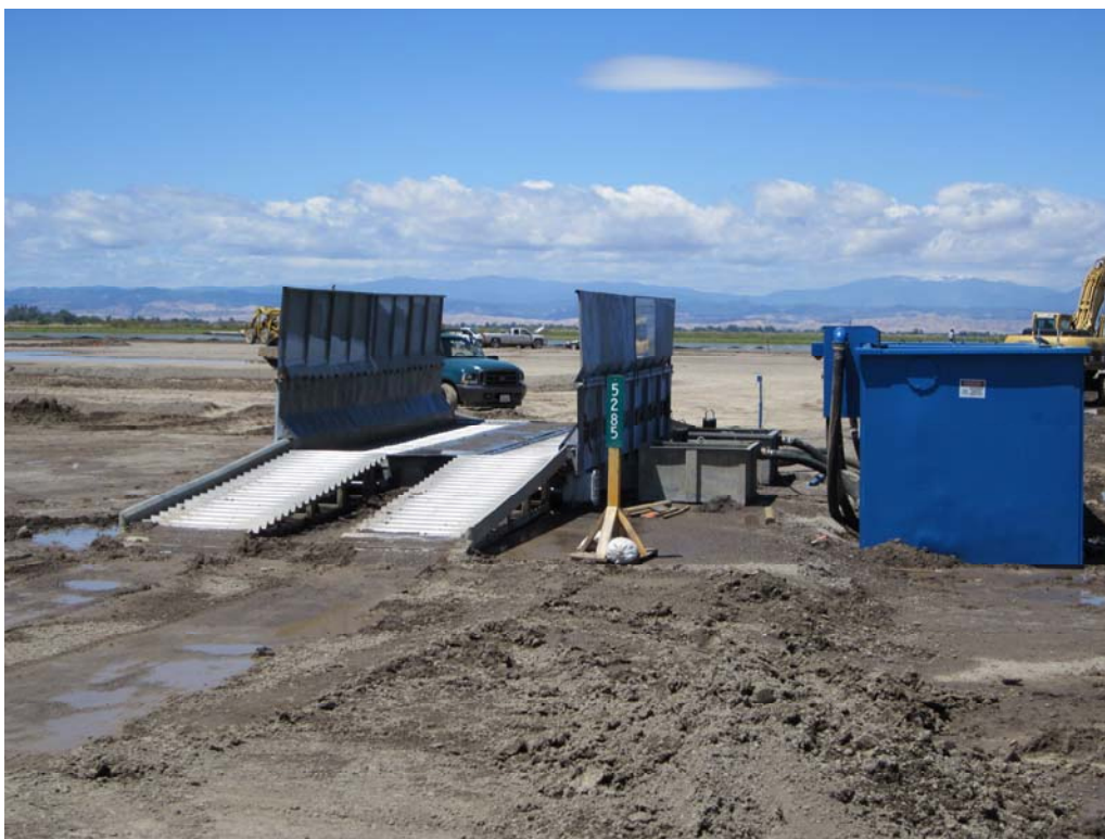
Photo 6: A tire washer and rattle plate are being utilized onsite for trucks exiting the compressor station site and entering McAusland Road in order to minimize track-out.
